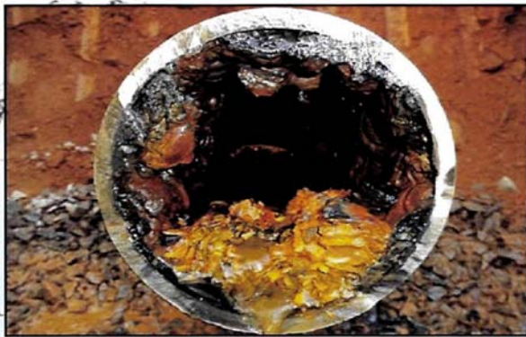
This project will allow us to replace antiquated and tuberculated pipes in our distribution system.
